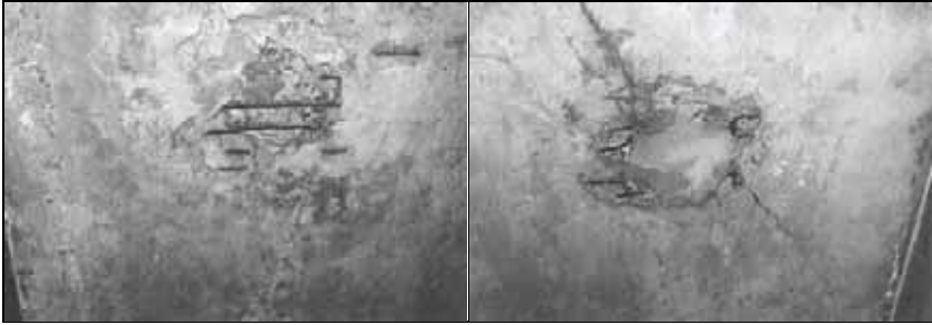
Figs. 25 and 26: Two of the four former openings through the roof of the morgue of Crematorium I in Auschwitz Main Camp, visible at the ceiling. They probably served as ventilation openings for the air raid shelter in 1944. They have been closed after the war “for museum purposes,” because their location makes it obvious that they couldn’t have served as Zyklon B introduction holes.
