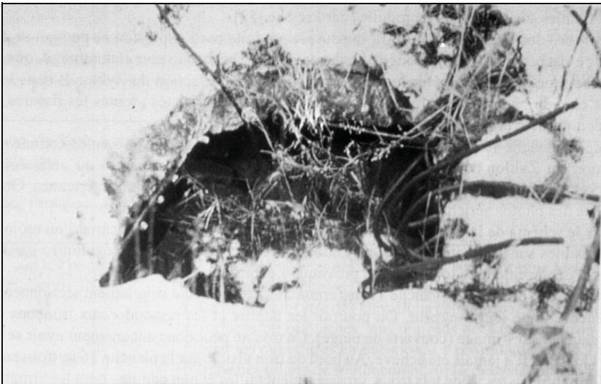
Fig. 45: Alleged Zyklon B introduction hole in the roof of Morgue 1 (“gas chamber”) of Crematorium II in December 1991. It is clearly visible that it was not cleared from the steel reinforcement rods. These were simply bent backwards.
