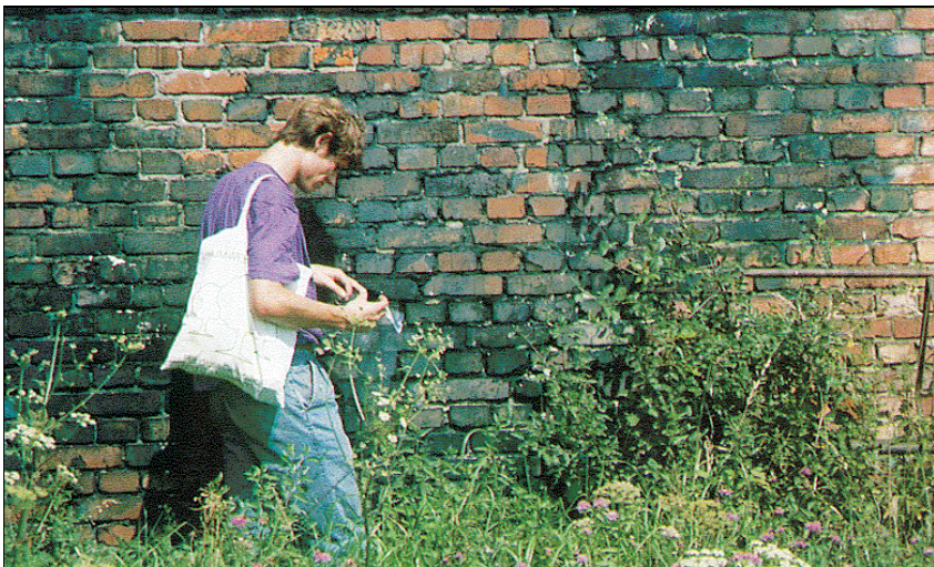
Fig. 71: In contrast to building 5a (see Fig. 68), the disinfestation wing of building 5b was used as a hydrogen cyanide delousing chamber for a longer period of time. Subsequently, the outside of its walls are covered with blue spots, unimpressed by 50 years of weathering here as well.
